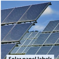
Solar panel labels
